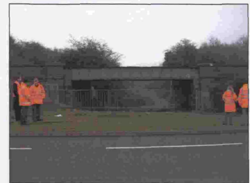
View Of Underbridge 9 (Looking East) Situated North of Proposed Location Bermuda Park Station (Feb. 2010)
